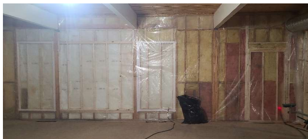
New window openings were framed and temporarily insulated while the windows are being manufactured.
