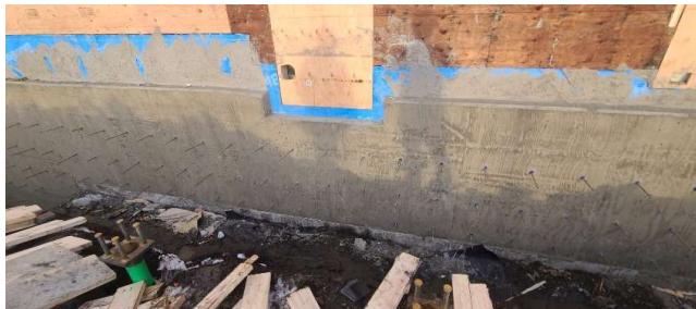
The completed concrete wall with a block out for the new door on the S side of the building.
